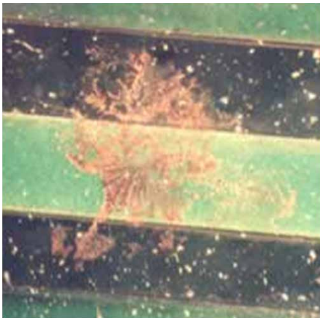
Figure 1: Condensation and conductive sediments can make up an electrolyte solution that under a DC voltage can lead to formation of a conductive path. Known as electro-migration, this process can lead to short-circuits or current leakage. The photo shows the migration of copper on a printed circuit board.
